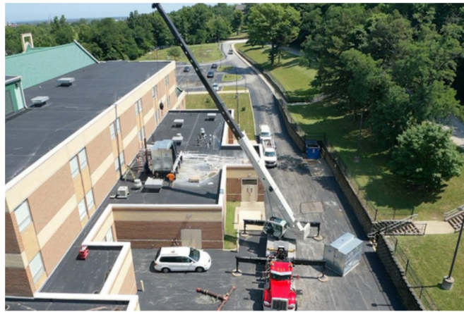
Above: Cranes move new chiller units into place on the roof of Kirk M.S.
